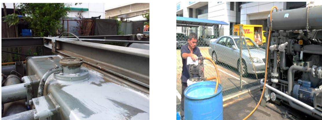
Figure 5-19: Engine coolant tank preserved with water mixed with VCI cooling additive
