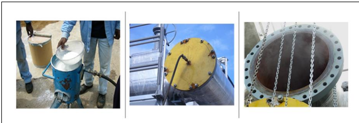
Figure 3-3: Use of VCI powders in offshore pipeline maintenance for hydro-testing and long-term storage.
