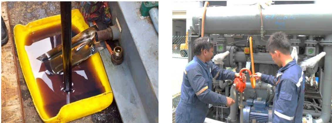
Figure 5-18: Drain out existing oil and re-fill with engine oil mixed with VCI engine additive
