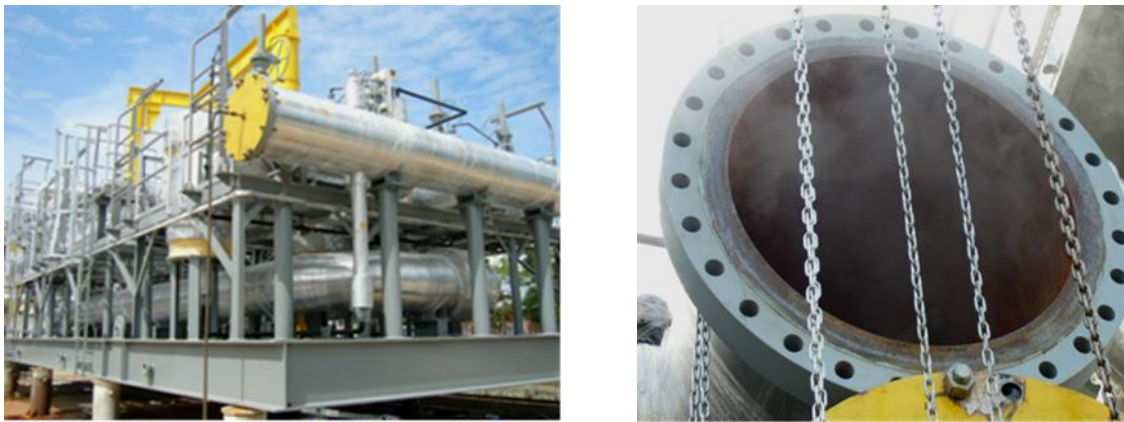
Figure 5-23: Preservation of piping system with VCI fogging powder
