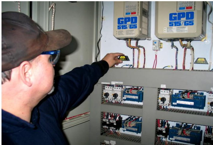
Figure 5-24: Application of VCI electronic spray, VCI electrical insulator, and VCI emitters in control panels
