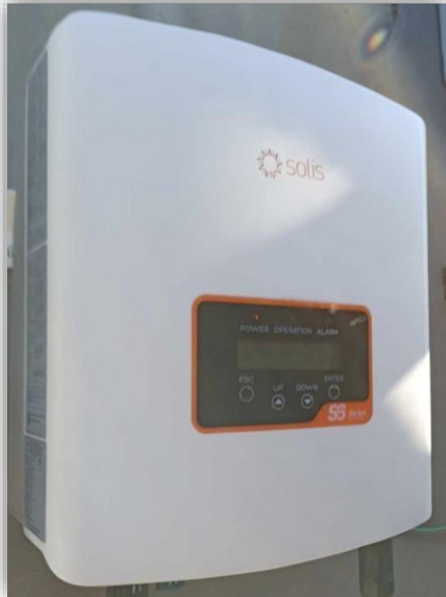
Figura 12. Inversor Solis 3.6 kW.
