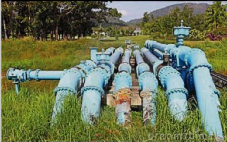
Painted steel water pipelines.
