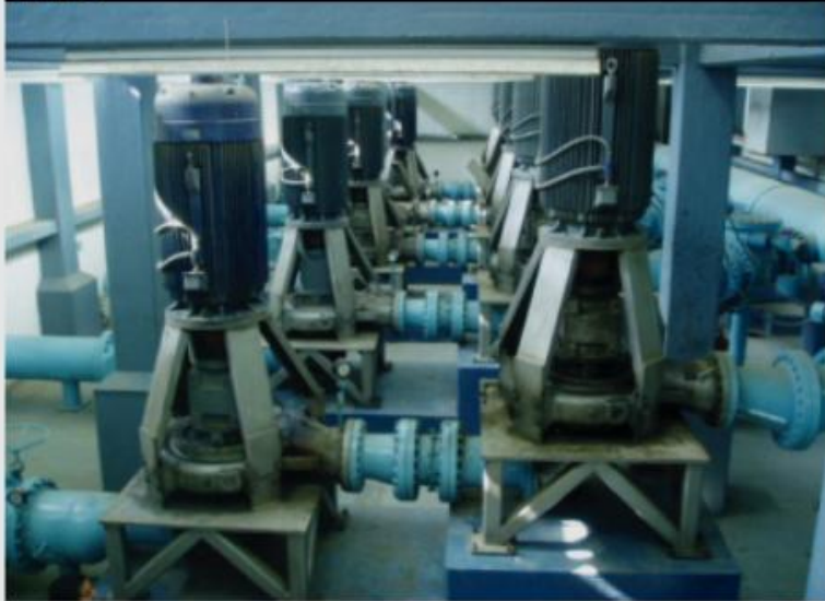
Pumps for water transportation.
