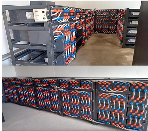
Fig. 2. Lead-acid battery bank
