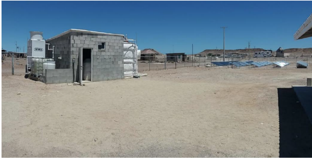
(a) Gabinete de control externo a Chiller LUCY
