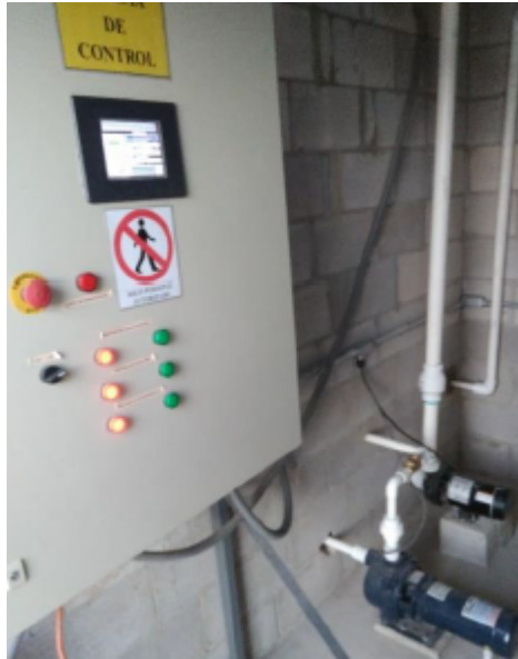
(a) Gabinete de control externo a Chiller LUCY
