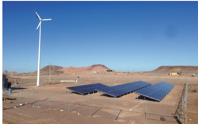
Fig. 1. Microgrid of the community of Puertecitos, Mexico.
