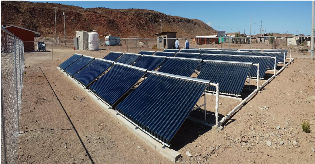
Fig. 1. Evacuated tube solar collector field.
